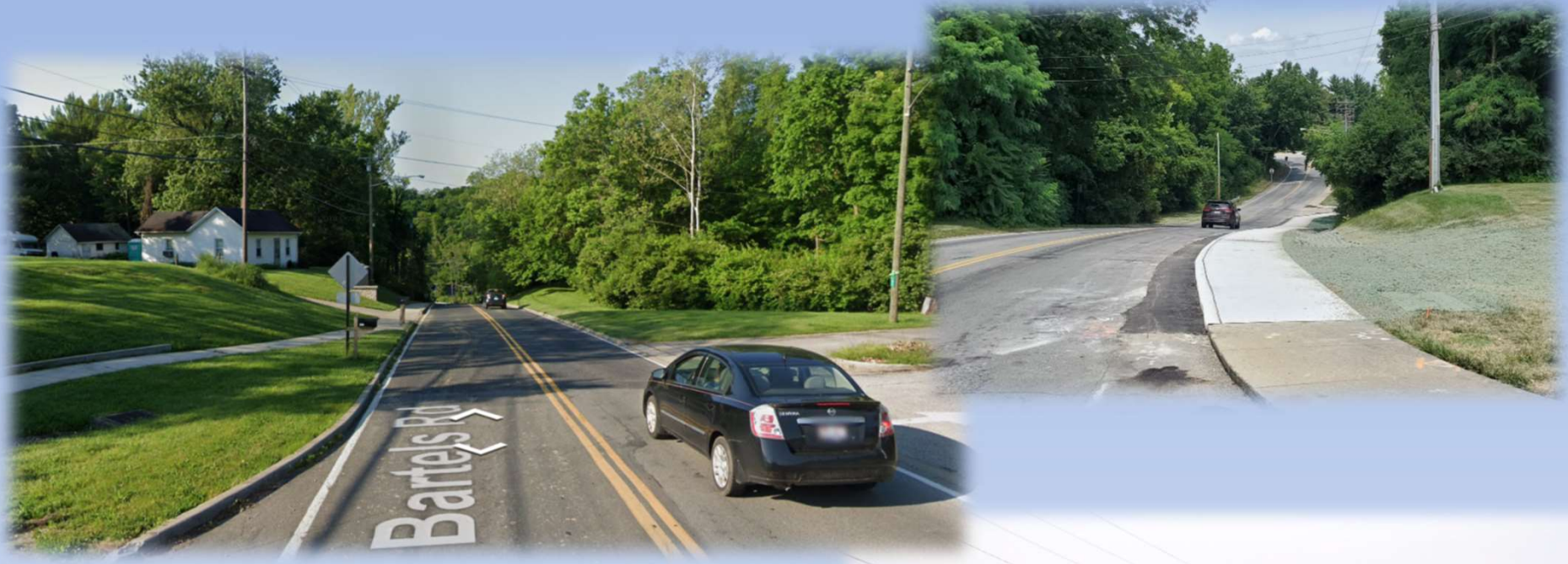
Installed sidewalk on west side of Bartels from Newtown Road to Clough Pike and resurfaced Bartels Road (Hill) with non—skid material
